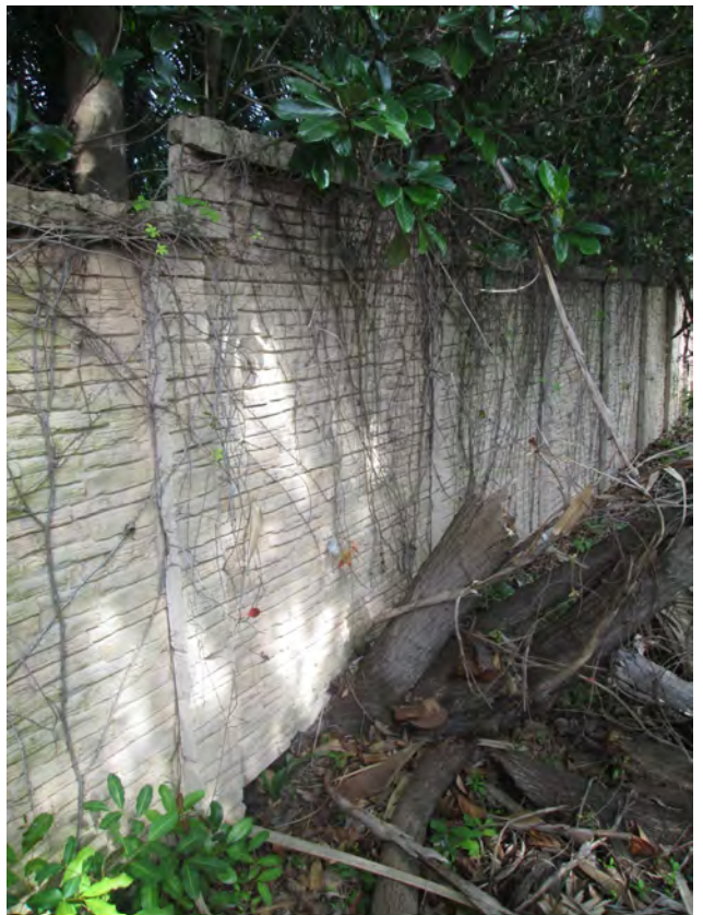
Vines growing on South Perimeter Wall
