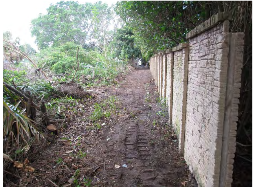
South side of South Perimeter Wall near west end – access for wall repairs
