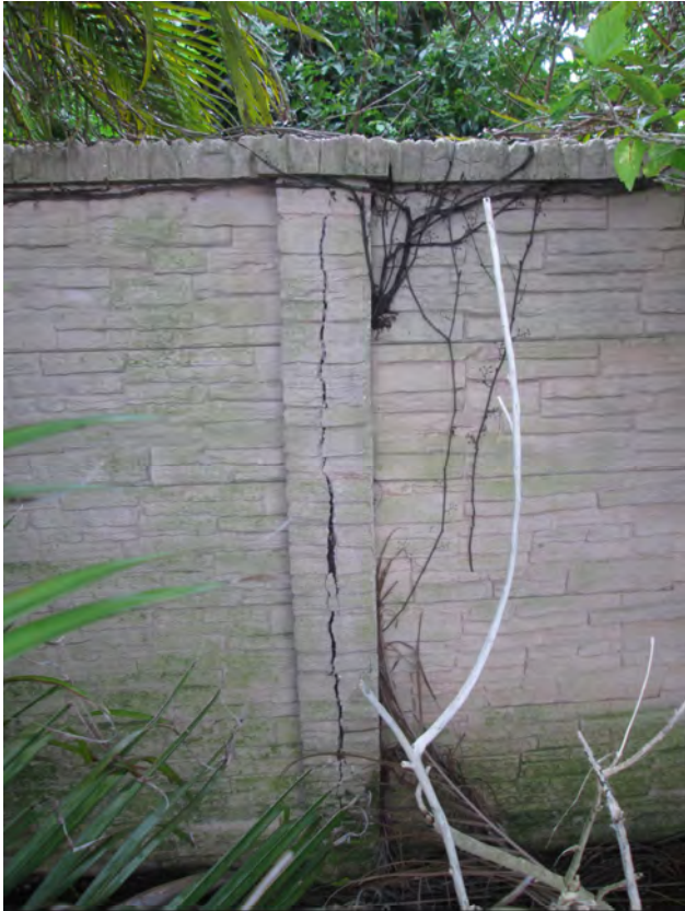
Vines growing on South Perimeter Wall
