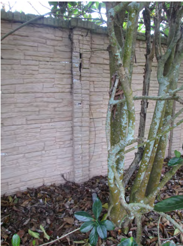
Vines growing on South Perimeter Wall
