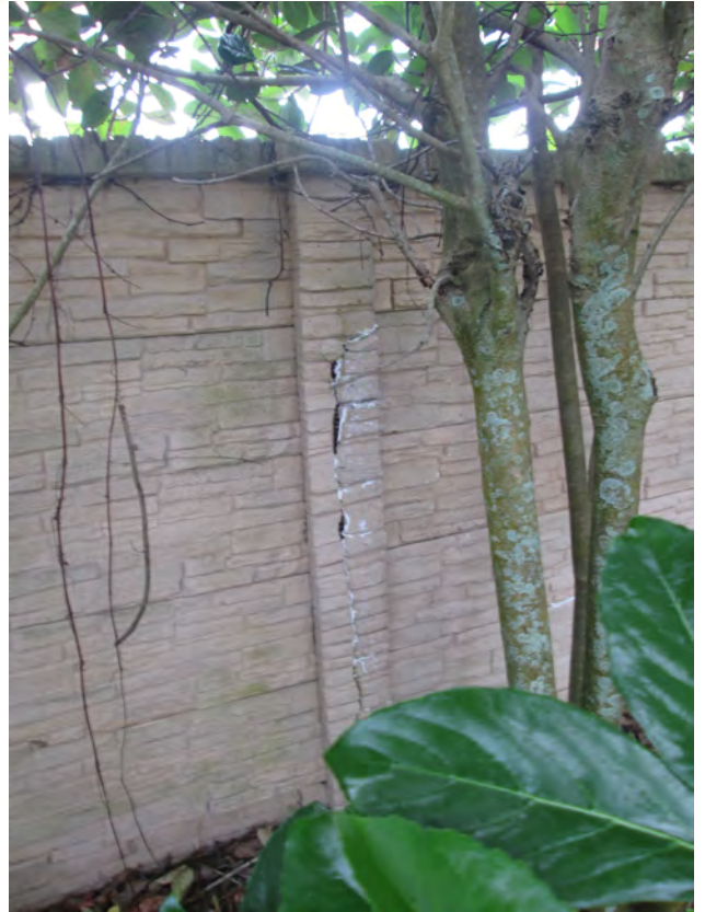
Tree limbs on South Perimeter Wall
