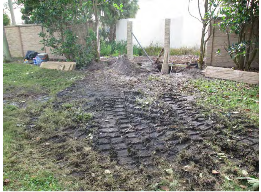
Minor lawn damage from Ligustrum removal and post replacements
